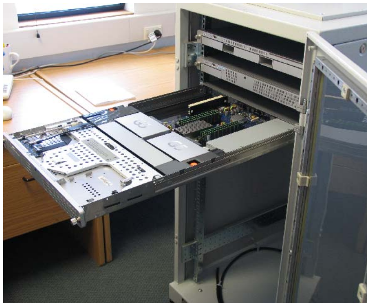
Figure 1: The 24-Unit Rack cabinet containing a partially constructed “Monte” dual-G5 compute cluster.
