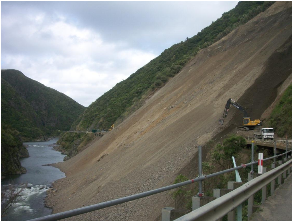
Figure 1.1 The Manawatu Gorge landslide photographed during remediation works. (Photo: Muhammad Imran, March 2012)
