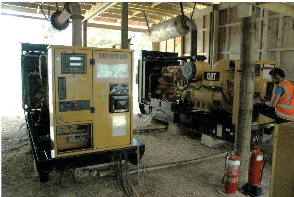
Figure 18 – Niue: Temporary Power House (following 2006 fire)
