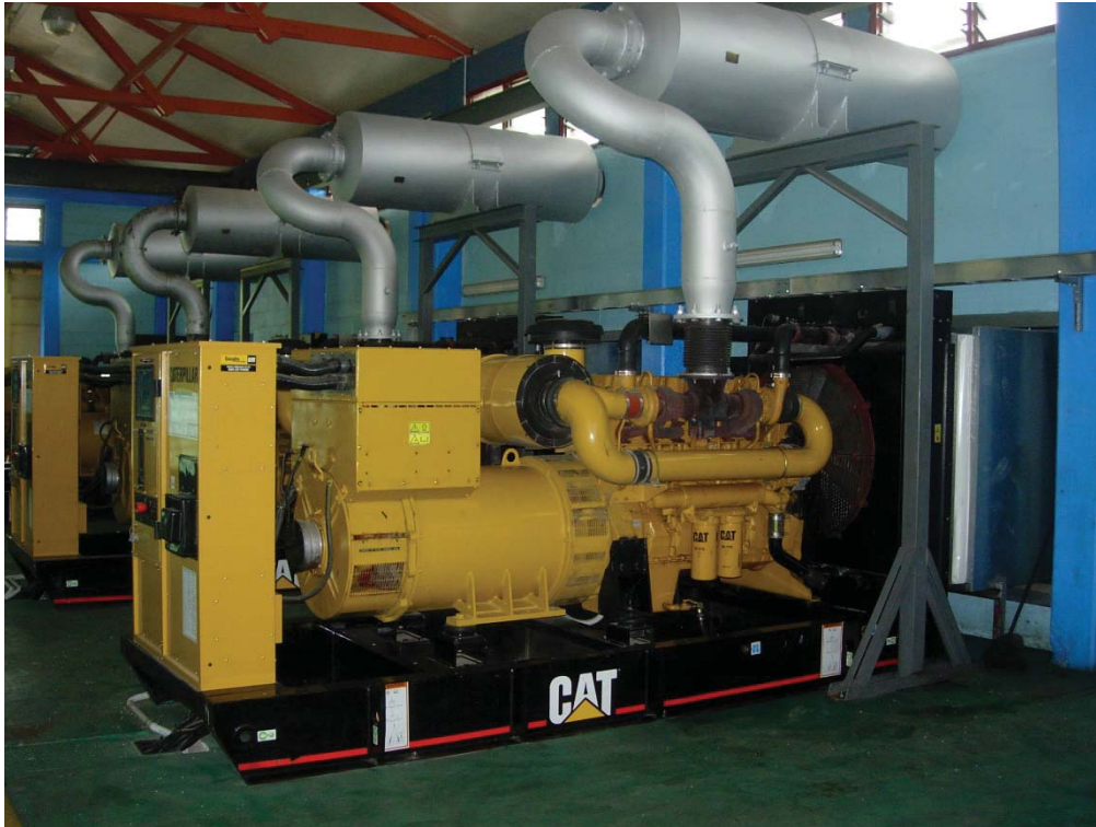
Figure 17 – Niue: NPC Power Station
