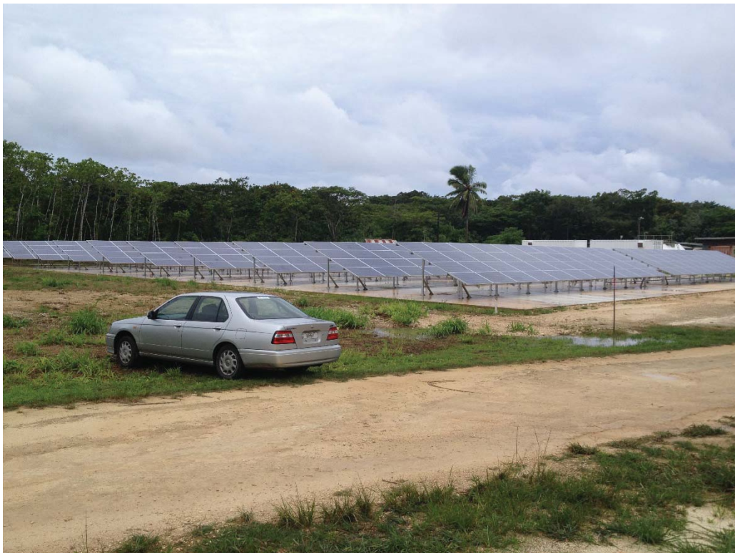
Figure 20 – 200 kWp PV Array at the Niue Power Station
