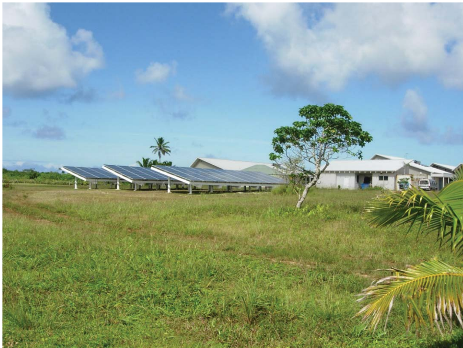
Figure 19 – PV Array at the Niue Hospital
